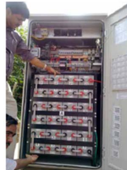
Figure 1: Alternating Mode: Smart Energy Controller & Cycling Batteries at VF-Essar Sites in India
