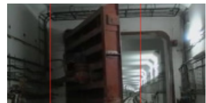
▲ Monitoring of civil air defense door intrusion
