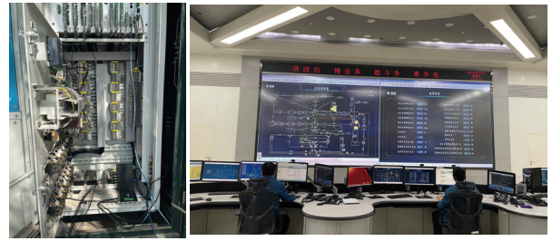
④ Real-time Sensing of Distribution Network via 5G RedCap
