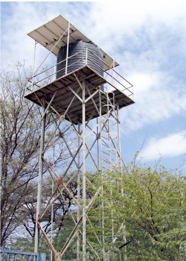
This previously installed, but inoperable solar water pump is an example of another potential anchor client that ASD considered powering as part of their business model.
